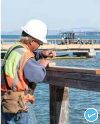
Paradise Beach Park pier improvements underway, upgrading 330 feet of aging wooden railing, concrete curbs, fish cleaning station, and trash cans.
