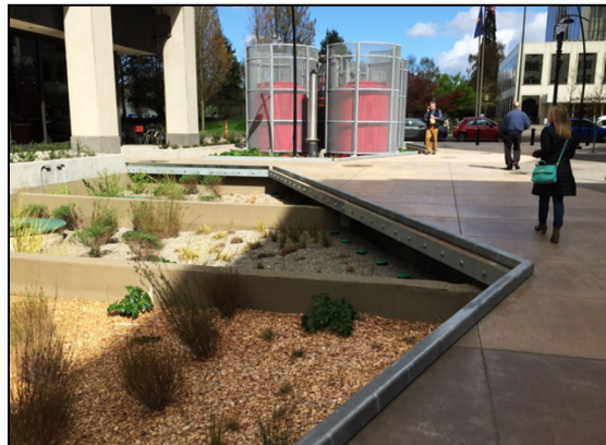
Figure 4: Example of trickling filters with an engineered wetland. From the Portland Hassalo on 8th project.
