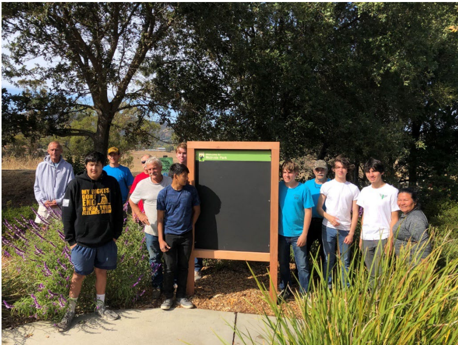
Above: Boy Scouts of America Troop 59 install a new kiosk and new landscaping, including mulching, at the McInnis Skate Park on October 17 th , 2021.
