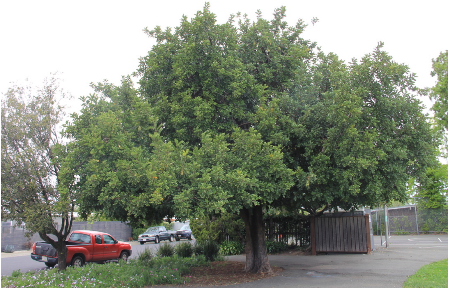
tree in question with visible uplifting of asphalt pavement nearby caused by roots
